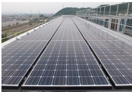
Solar panels at the Minase Research Institute
